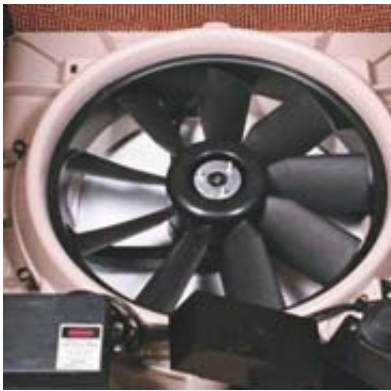
The inside of a Commercial Air unit
